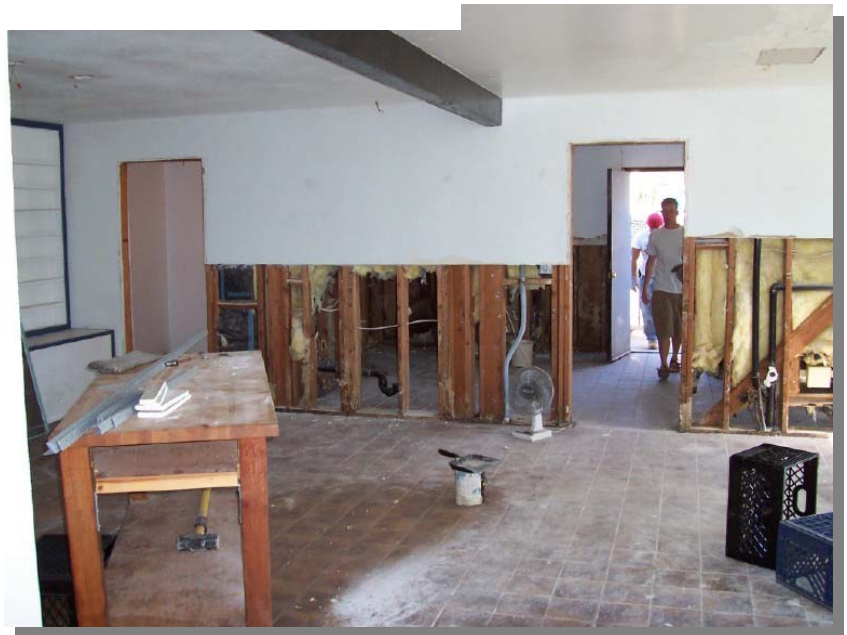
Looking towards the kitchen from the dining room. Lower portions of walls and insulation were removed due to mold.
