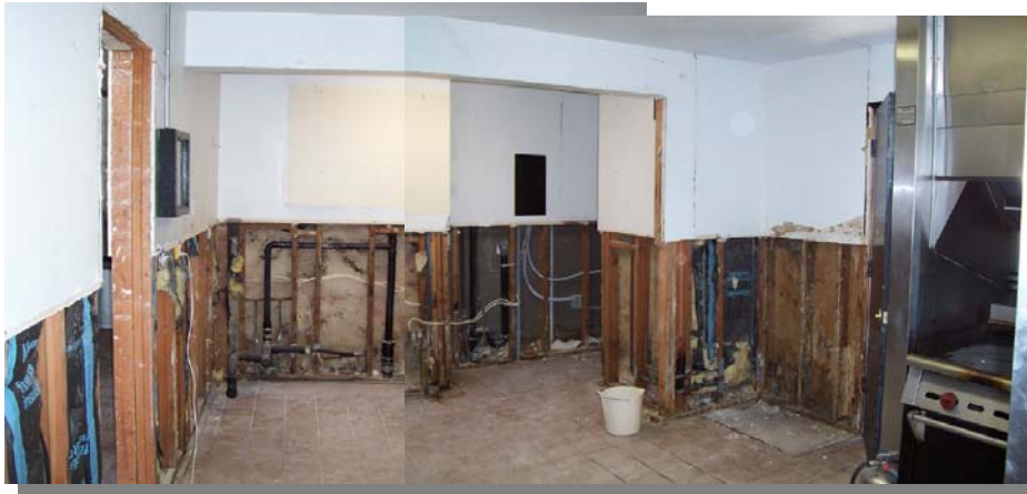
Panorama looking at back wall of kitchen, stove to the right, dining room to the left. Floor of the kitchen received a drain and slope to prevent further mildew and mold issues.
